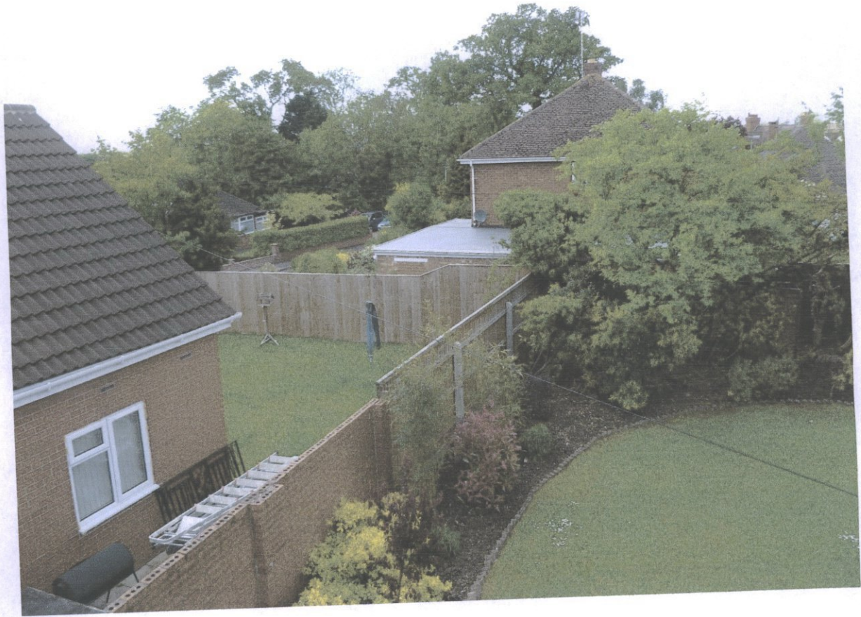
Photograph 2, showing absence of upper and lower guttering end caps
